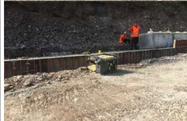
Power generator without drip tray, workers without PPE
